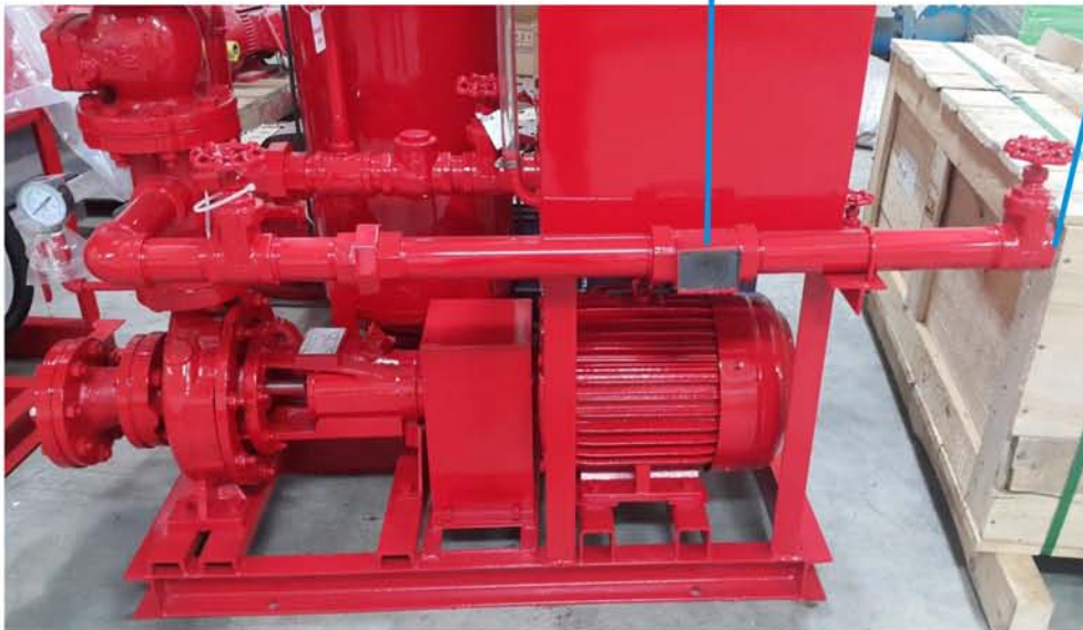
Installed discharge pipe on Flow Meter pipeline, to drain water when testing flow
